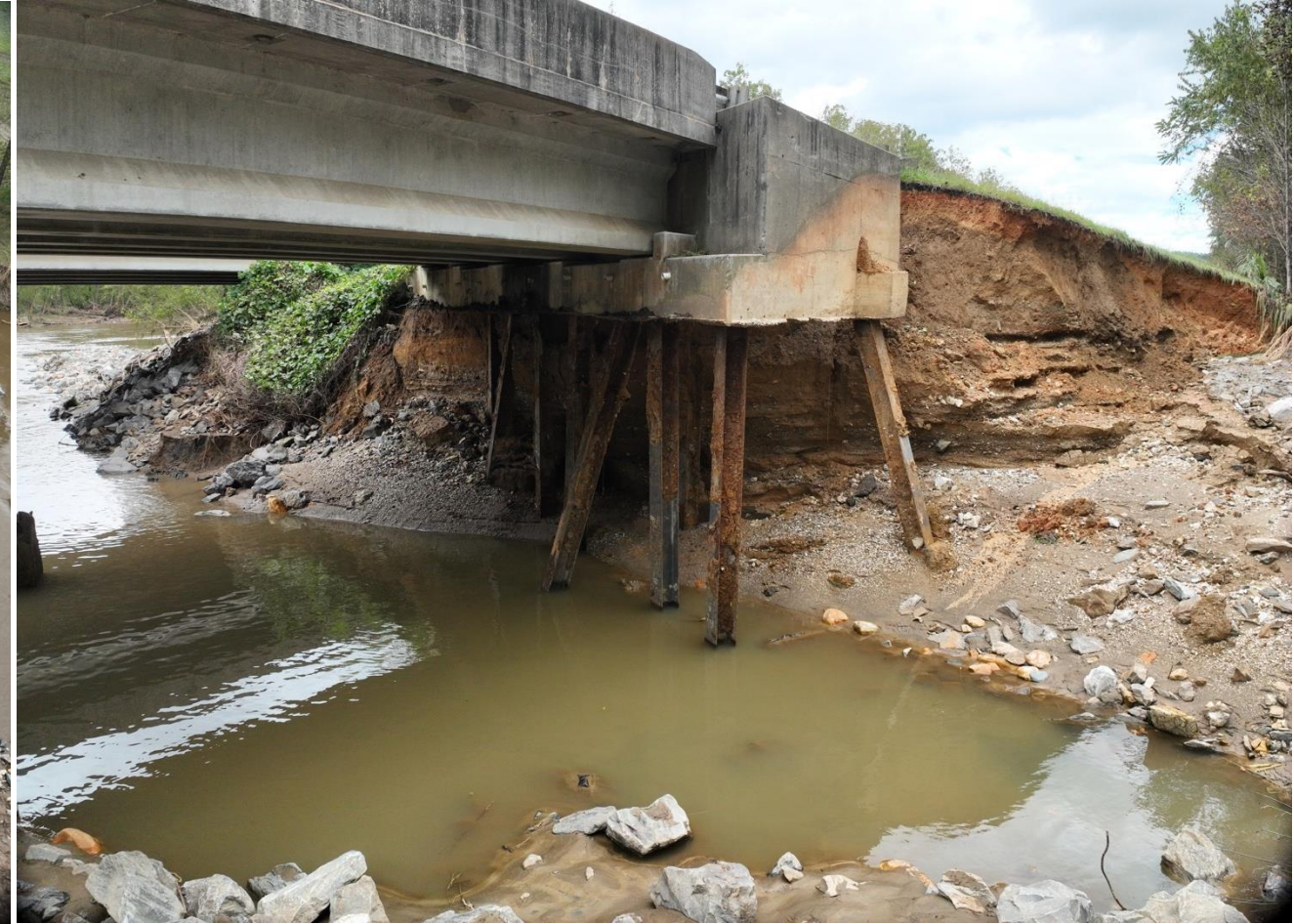
Aviation, Structures and TSMO unit coordinated to further inspect, then reduce lanes for safety
